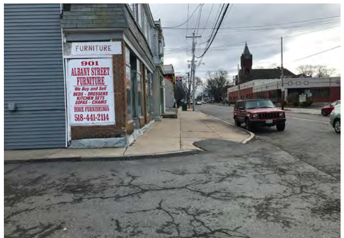
Several intersections are lacking in ADA curb ramps and crosswalk striping. This photo was taken between Steuben Street and Craig Street.
