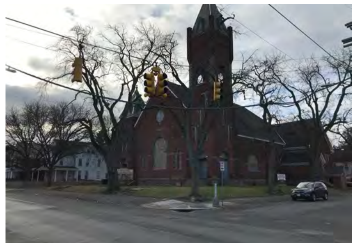
There are some ADA cross ramps that have been added recently, but most intersections do not have crosswalk striping and the curb ramps often lead to sections of sidewalk that are no longer accessible due to their condition. This photo was taken at the Steuben Street intersection.
