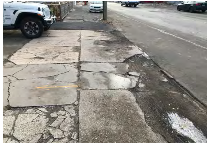
In some area, the road has been paved higher than the sidewalk, and when combined with the poor condition of the sidewalk, this leads to drainage conflicts and pooling of stormwater in walking areas. This photo was taken on Albany Street between Brandywine Avenue and Steuben Street.
