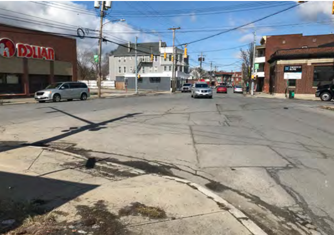
There is an ADA access ramp at the point of the property between Crane and Chrysler, but it leads to the center of the intersection, encourages maximum length and exposure crossings, and there is no crosswalk striping at the intersection.
