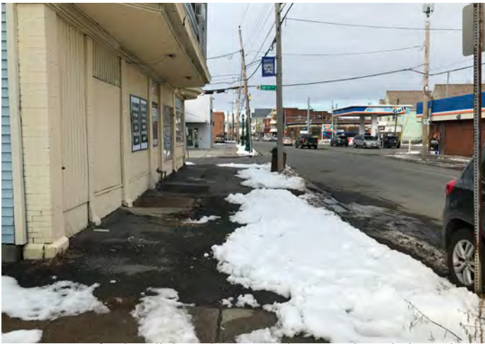
Many areas of sidewalk have been paved over with asphalt as shown here at the 6th Avenue intersection.
