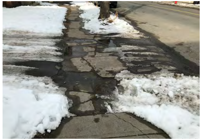
Many of the driveway transitions are in poor condition and make sidewalk use difficult for anyone with walking challenges or pushing a stroller. This photo was taken between Main Avenue and Ostrander Place.
