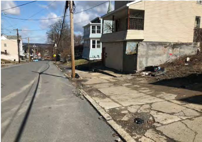
Large portions of the sidewalk are in poor condition, particularly where cars are parking and driving on them. The curb reveal is also largely absent in many locations. This photo was taken in the area between Bridge Street and Broadway.
