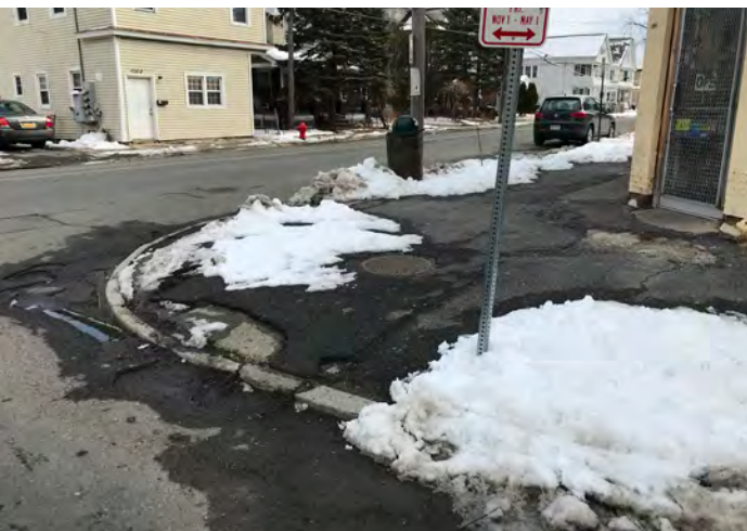
Many intersections are lacking ADA curb ramps and striped crosswalks as shown here at the 6th Avenue intersection.
