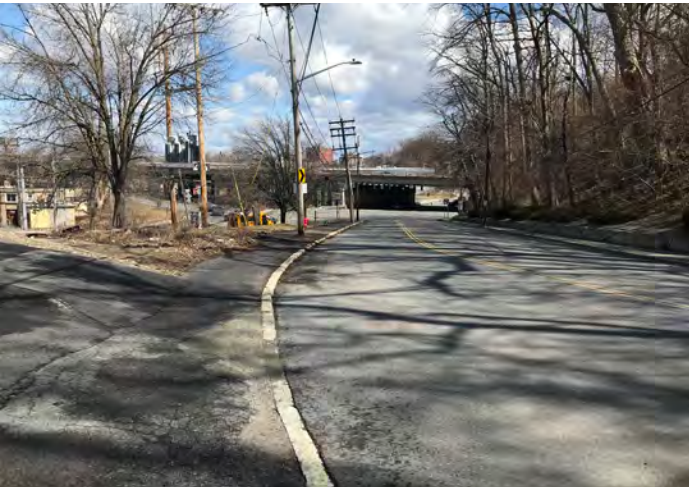
In some areas between Bridge Street and Broadway, private owners have paved over the sidewalk with steep areas of asphalt as a way to reduce the slope in their driveways. This makes the cross-slope steep and difficult to navigate, particularly in precipitous weather.
